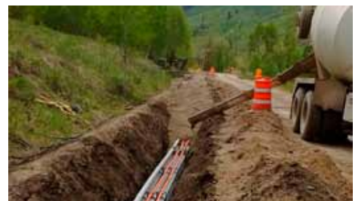
Summer weather provides opportunity to get critical work, like the Telluride/Mountain Village Reliability Project installed and online.
